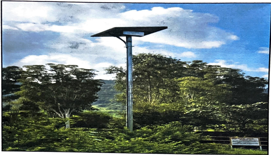
Figure 7: Solar Street Light
